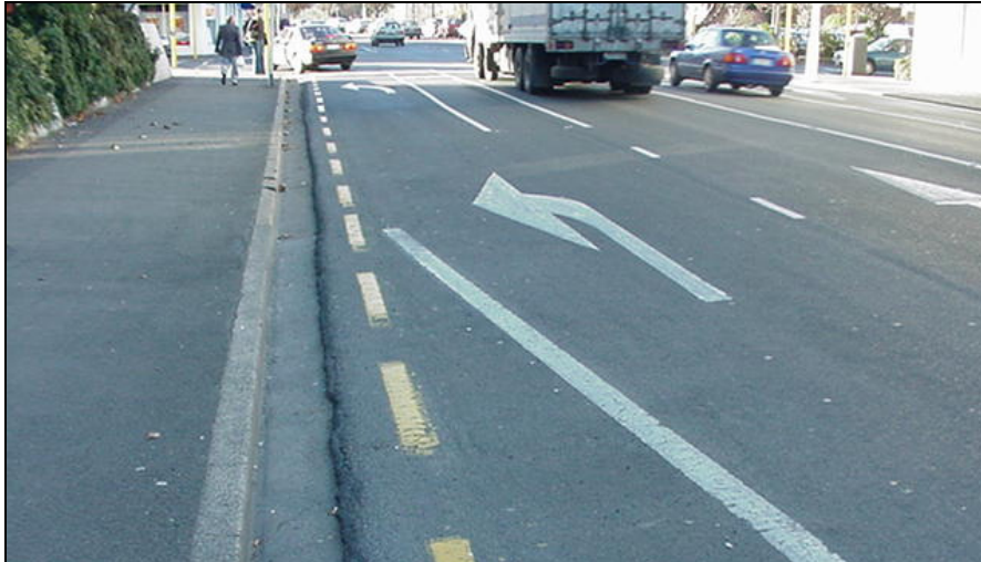
Photo 2: Excessive build-up of asphalt presents a potential hazard to cyclists
